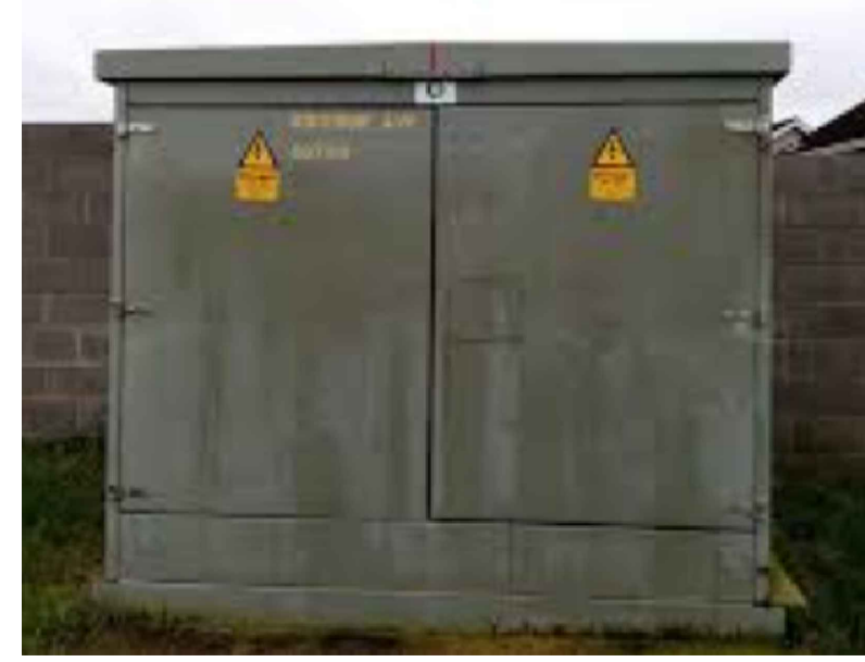
TYPICAL SUBSTATION KIOSK
